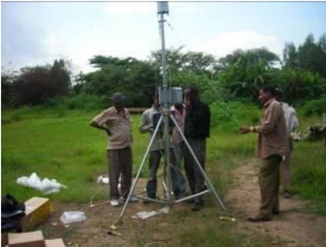
Figure 7 Automated met station installation
